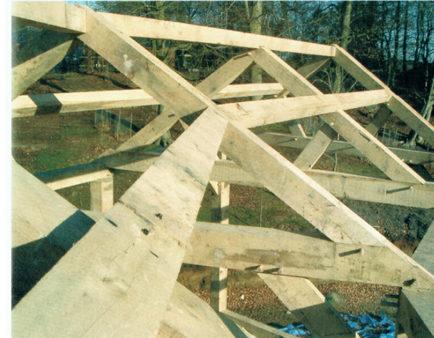
Above left and this page: the joints were traditional mortice and tenon – but 90° angles were few and far between
